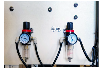
Air pressure controls
